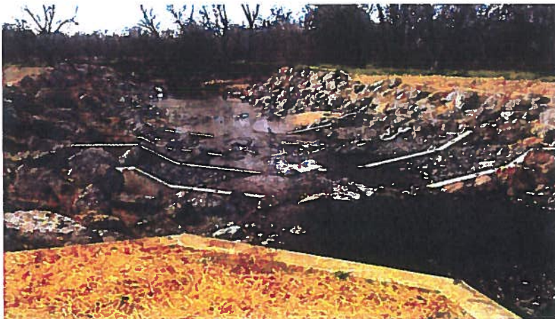
Fish Passage system installed at Lincoln Gauging Station.
